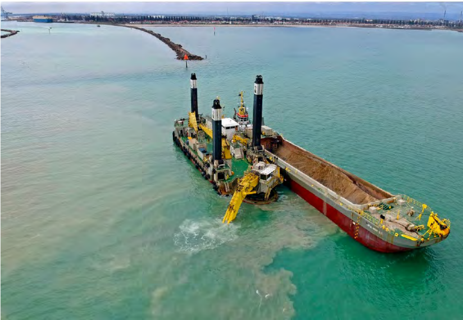
Photo 11 Backhoe Dredge Magnor widening the shipping channel at Port Adelaide River mouth (Source: Boskalis 2020)
