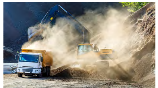
Figure 29 Example of dust generation caused by earthworks (Source: Stratec 2021)
